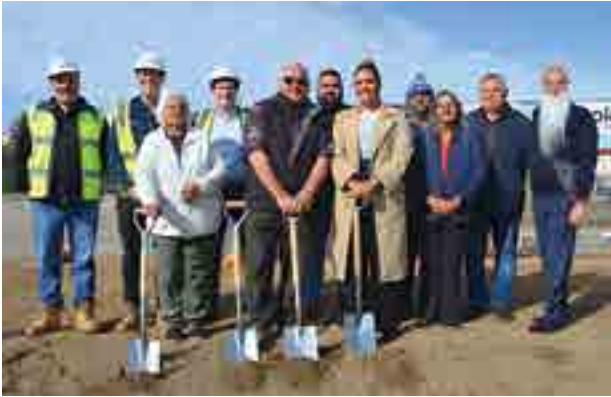
Contractors join Val Rigney, Steve Sumner, Tahlia Lloyd, Lawrie Rankine, Ellen Trevorrow, Derek Walker and Alfred Agius as work begins at the former Lower Murray Nungas Club. Photo: Peri Strathearn.
